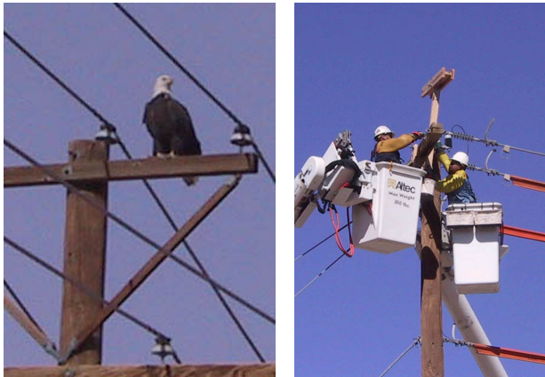
(L) Rio Bosque's wintering Bald Eagle, (R) El Paso Electric personnel install perch on pole near Park.
