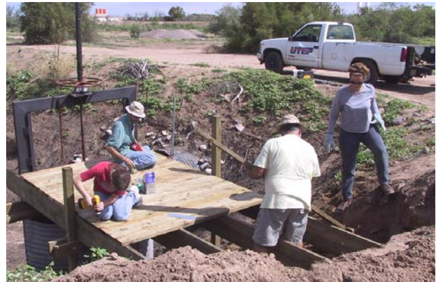
Friends of the Rio Bosque rebuild the walkway to Water Control Gate 1 on Aug 19, 2006.
