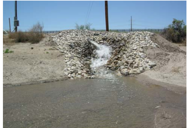
The new well at the park's inlet in operation, April 29, 2009.
