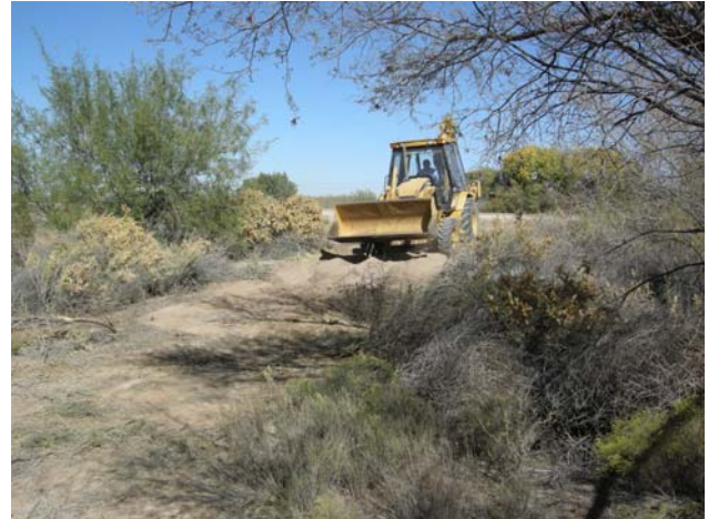
The USIBWC begins work on the channel that will connect a turnout on the Riverside Canal with Rio Bosque's main channel, November 13, 2012.
