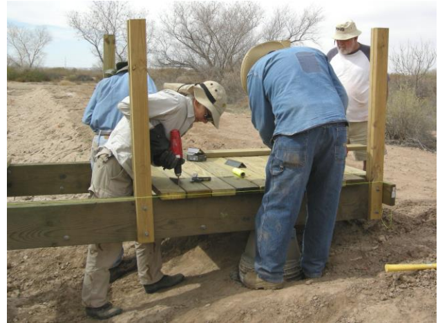
Friends of the Rio Bosque build a footbridge over the water-delivery channel from the planned turnout on the Riverside Canal, March 18, 2013.
