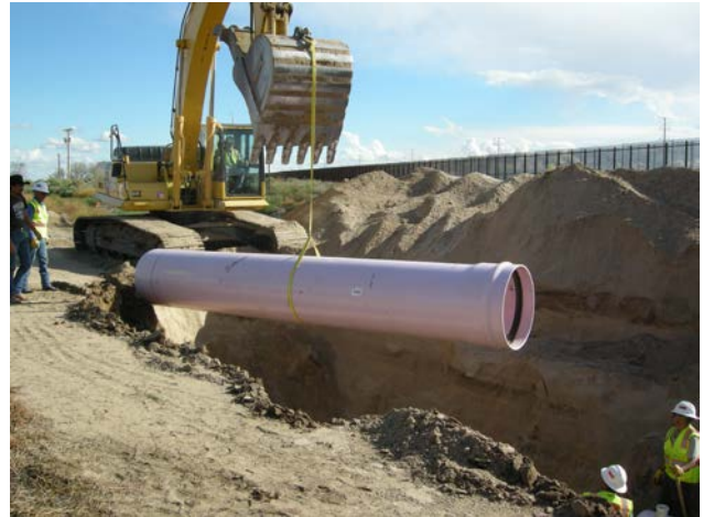
Pipeline construction at Rio Bosque, Oct 20, 2014. El Paso Water Utilities completed the final segment of the pipeline in March 2015.
