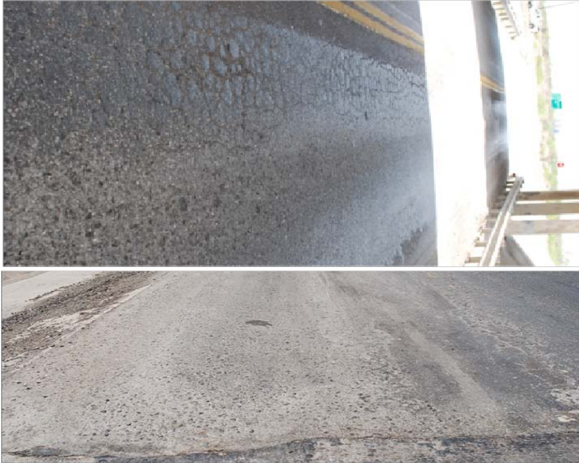
Figure 7.14 – Alligator cracking and Surface Rutting along US 83 Underpass.
