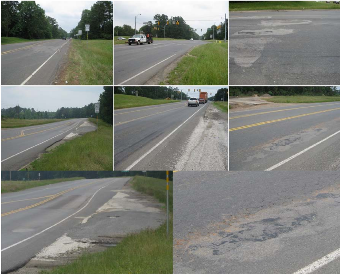
Figure 7.2 - Views of the Conditions of SH 315 and SH 149 Intersection.
