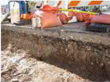
Location (D): 5 th street south of intersection
