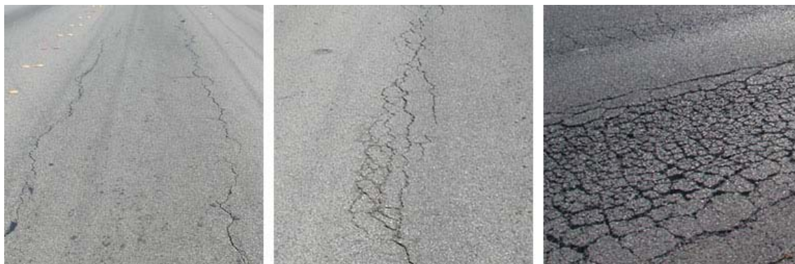
Figure 2.7 - Fatigue or Alligator Cracking on Asphalt Pavements.
