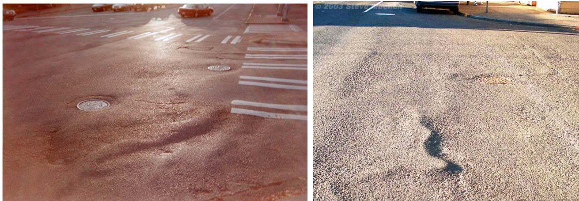
Figure 2.6 - Shoving on Asphalt Pavements.
