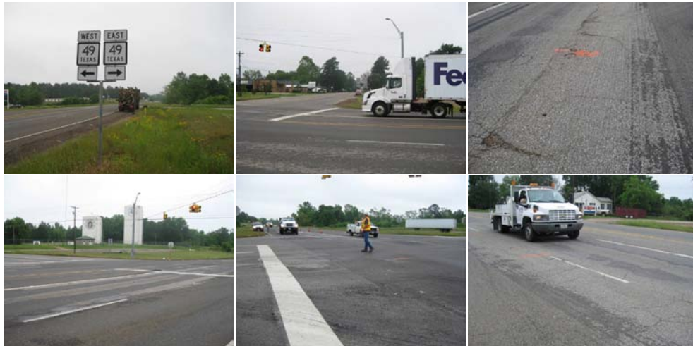
Figure 5.4 - Views of the Conditions of SH 155 and SH 49 Intersection.
