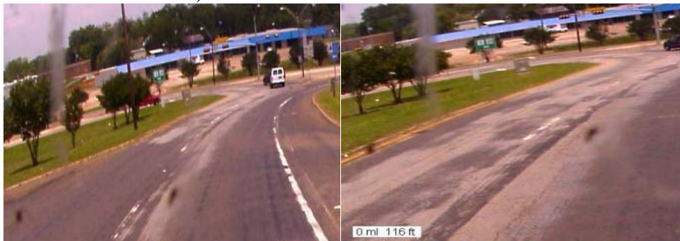
b) US 259 Northbound Outer Lane
