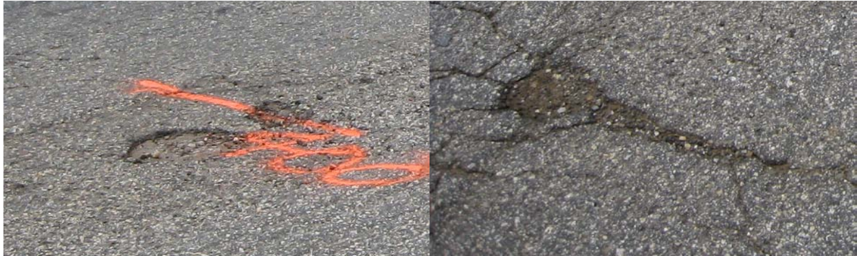
Figure 5.6 - Cracking Resulting in Potholes on SH 49.
