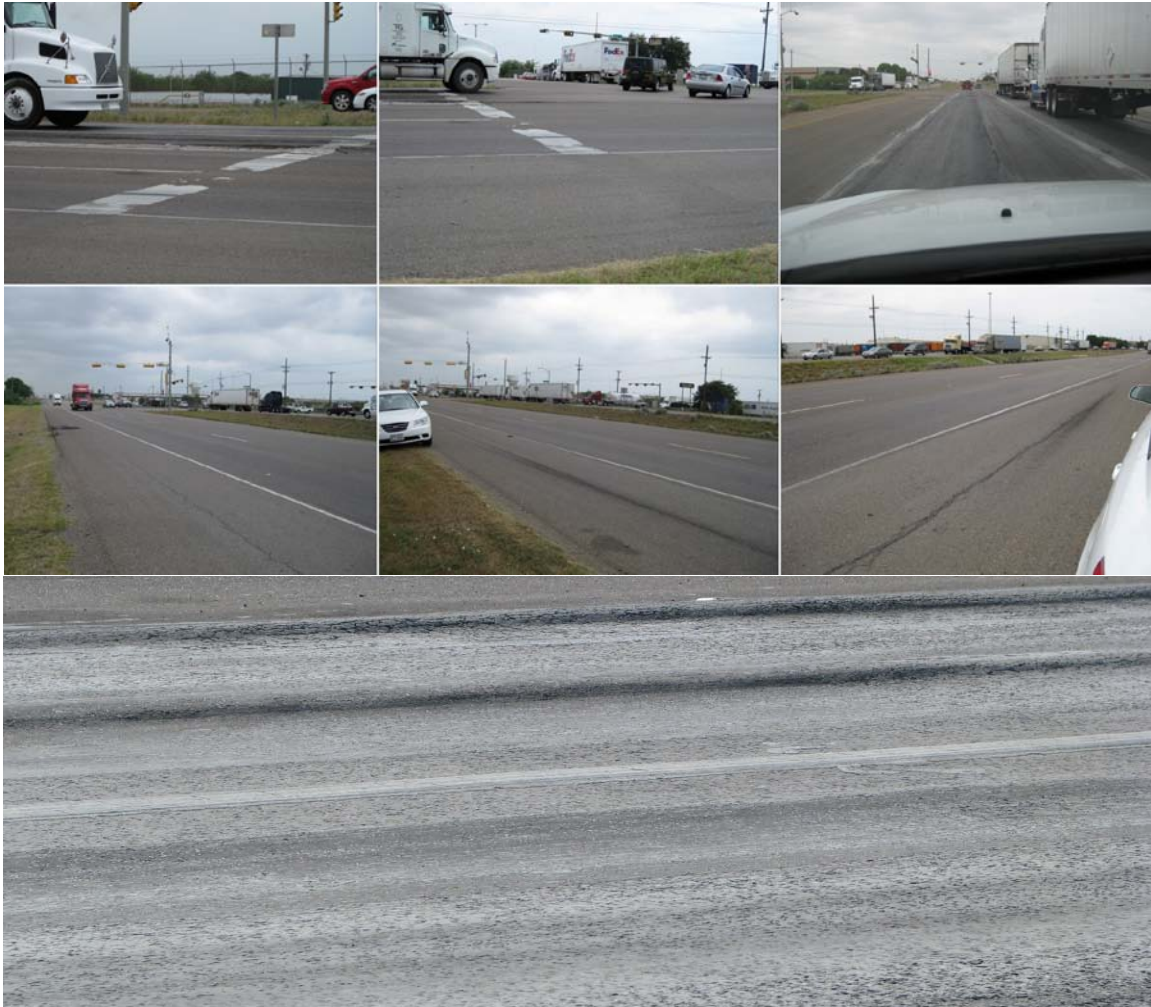
Figure 7.11 - Views of Conditions of Intersection at FM 1472 in Laredo District.
