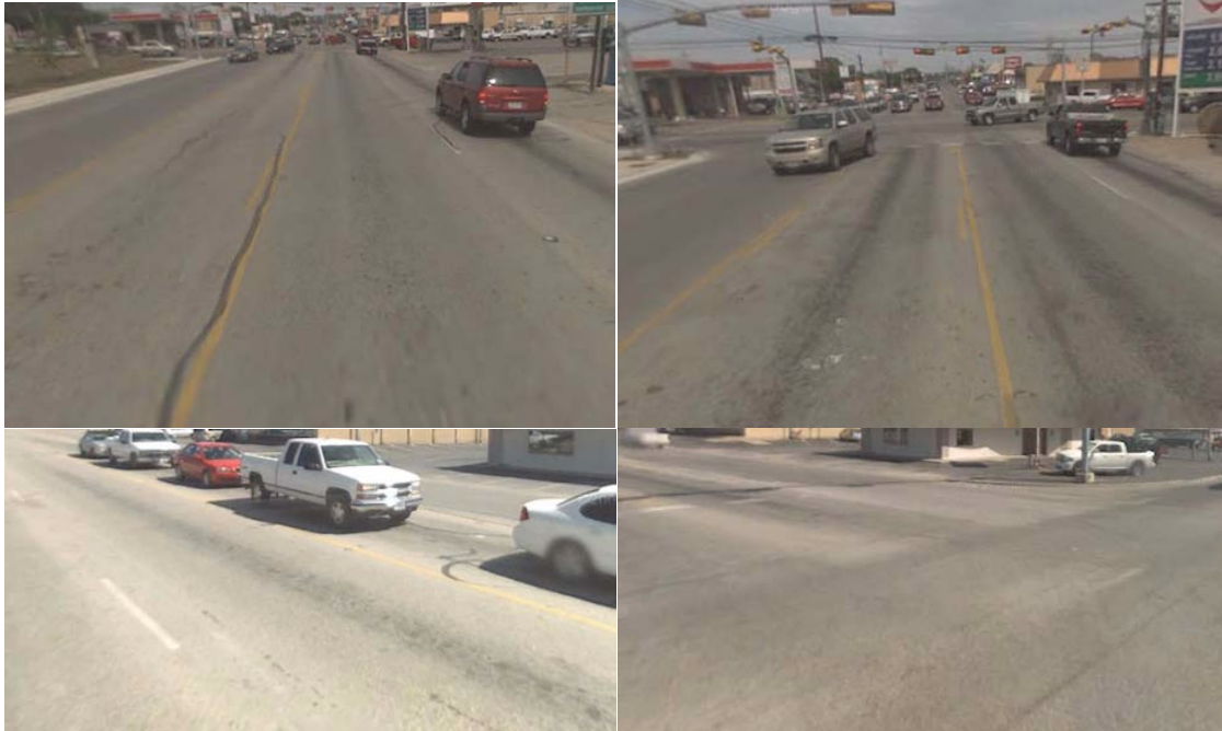
Figure 7.6 - Conditions of US 281 and SH 29 Intersection.
