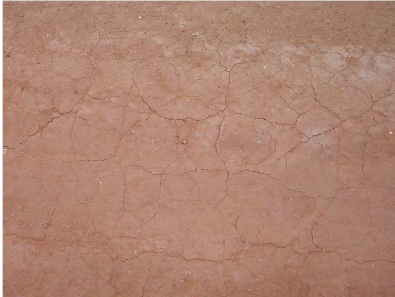
Figure 6.18 – Surface Cracking after 3 Days of Curing
