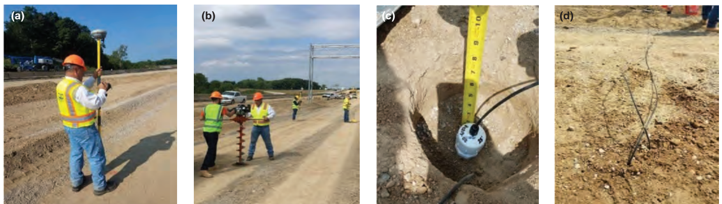
Figure 7-6. Installation process of embedded geophones: (a) GPS localization, (b) drilling with auger, (c) embedding ground sensors, and (d) wiring of geophones to data acquisition system.
