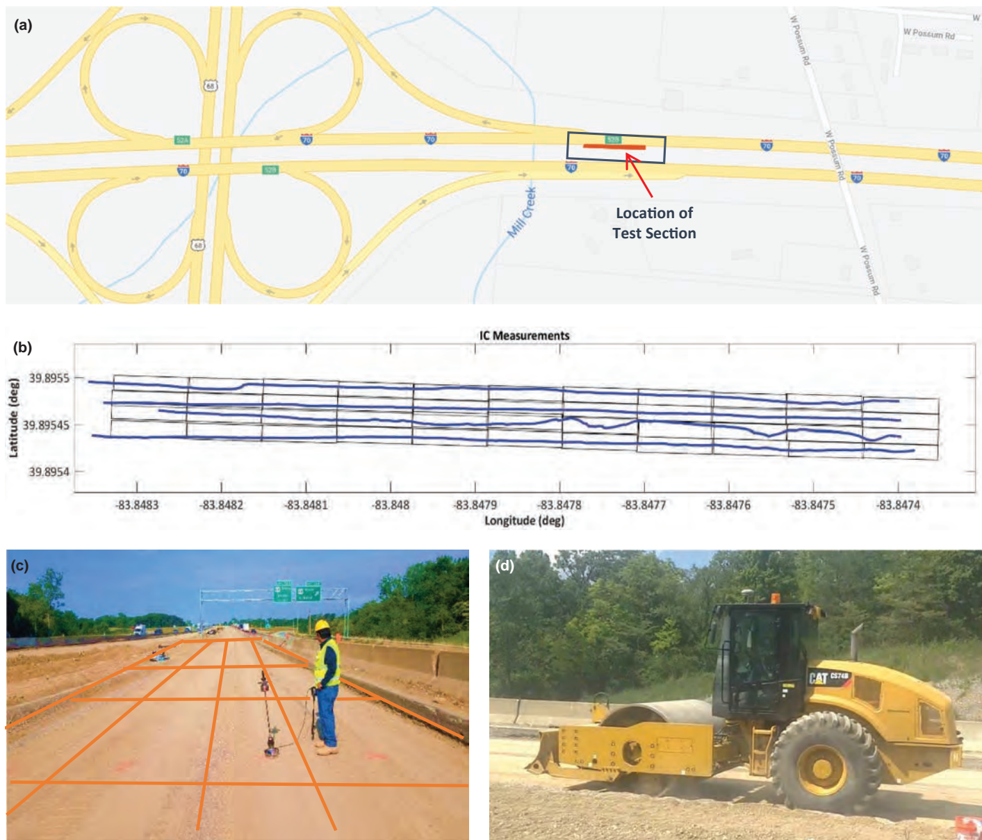
Figure 7-4. Overview of I-70 westbound reconstruction in Springfield, Ohio, showing (a) location of test site, (b) line passes during proof mapping of subgrade, (c) test section with sublots, and (d) roller during proof mapping of subgrade.
