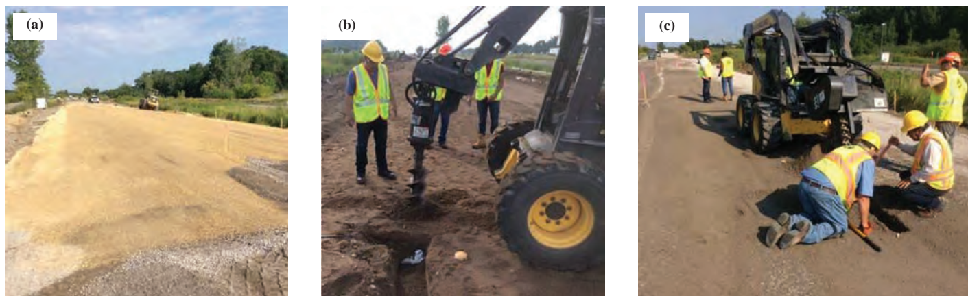
Figure 4-4. The MnROAD test strip: (a) a view of the test strip, and (b) and (c) UTEP and MnROAD personnel preparations for embedding ground instrumentation.
