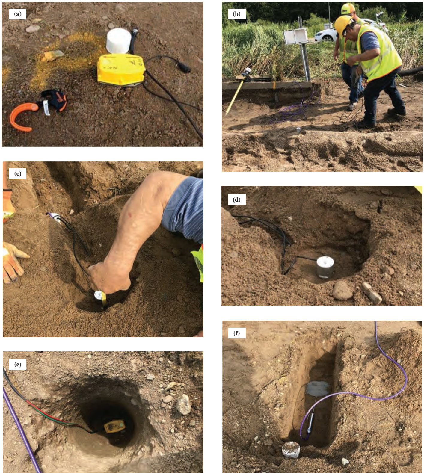
Figure 4-5. Installation of ground sensors: (a) preparation of ground sensors, (b) wiring of sensors by UTEP and MnROAD personnel, (c) embedment of geophone, (d) and (e) geophones within geomaterial, and (f) pressure cell within geomaterial.
