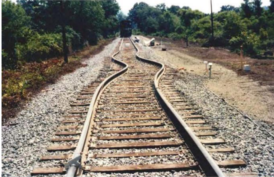
Figure 24. Example of Railroad Buckling [41]
